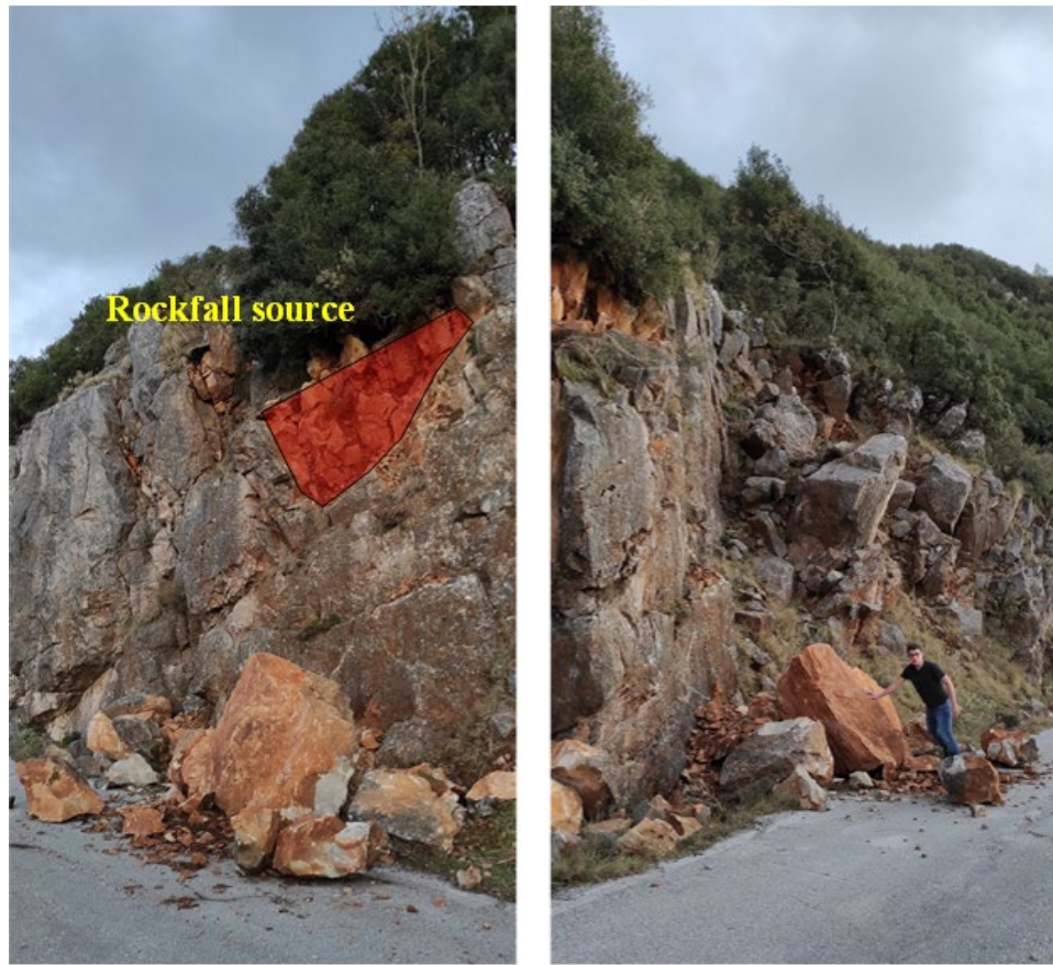
Figure 6.24. Rockfall in Cephalonia island ( 38.36995197^{\circ}\text{N} , 20.5684499722^{\circ}\text{E} )
