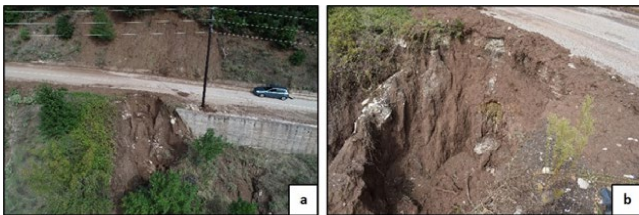
Figure 6.16. Rotational slide towards Porti village (39.425833°N, 21.665556°E)
